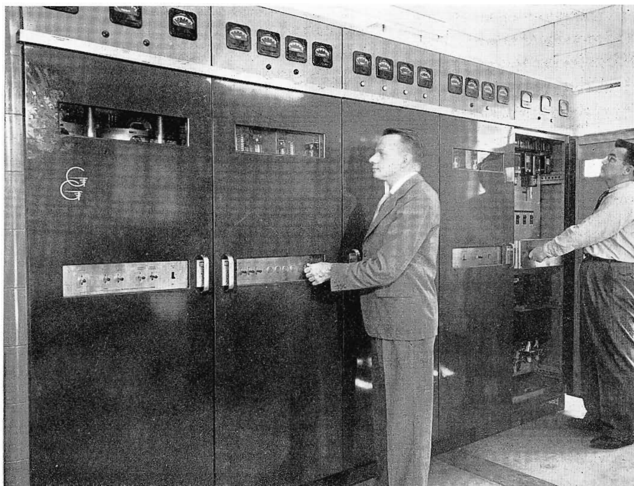
FIG. 9. The RCA BTF-10B Transmitter with Chief Engineer Thomas Phillips, left and Engineer Washington Elitchco.
