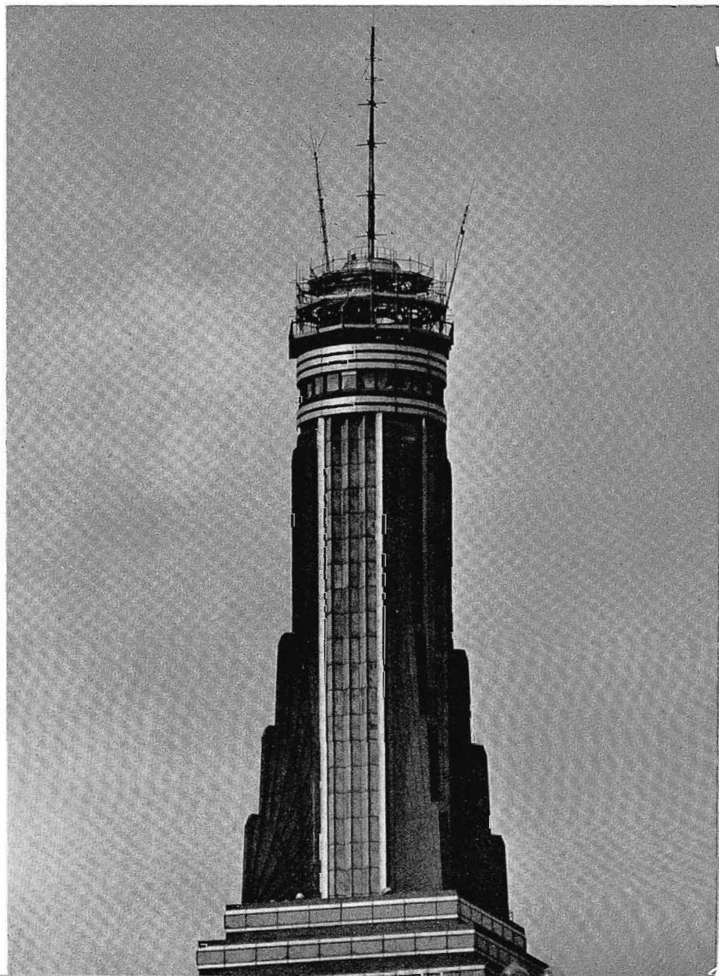
FIG. 1. View of the top portion of Empire State building showing temporary antennas located at each side. Note that photo was taken before old 67-foot TV antenna (center) was taken down. The three platform working levels provided are visible. Photo was taken from the Metropolitan Life Insurance Building with a 40-inch telescopic lens.
