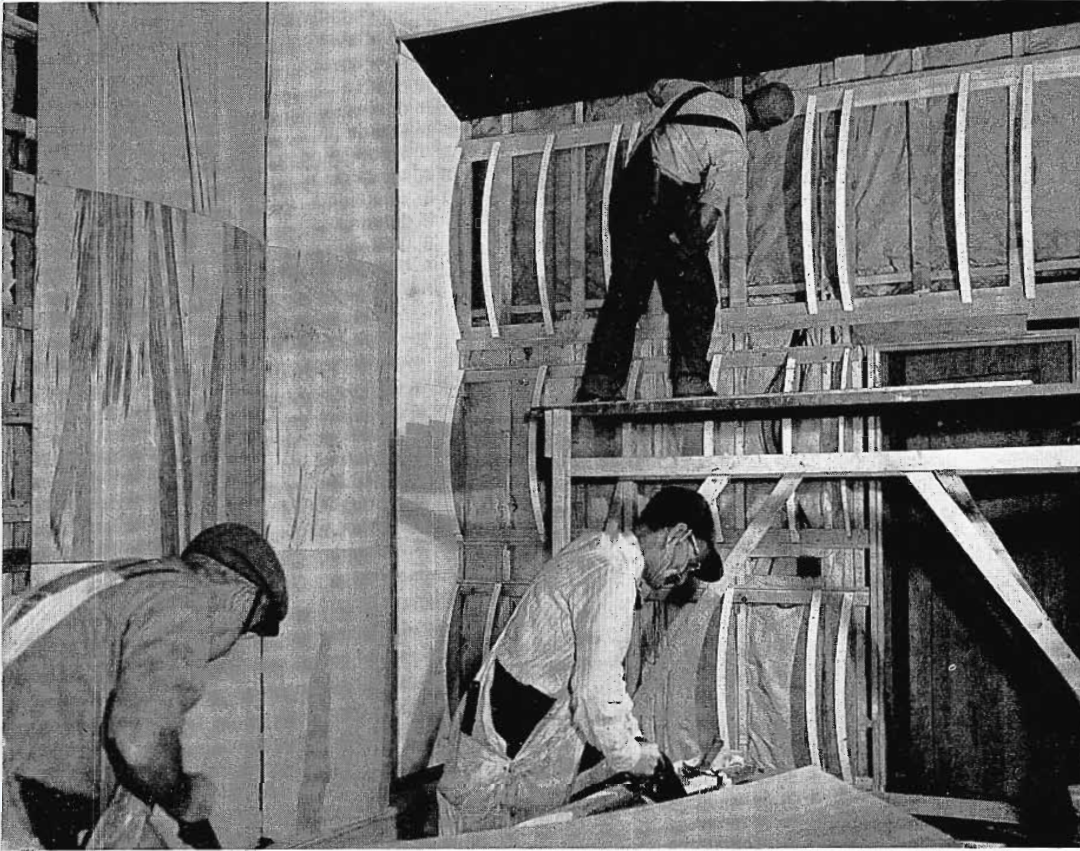
Studio B pictured during installation of acoustical treatment Roll insulation, the cylinder forms and fibre-covered cane ribs at right were covered with finished cylinders as shown at left.
