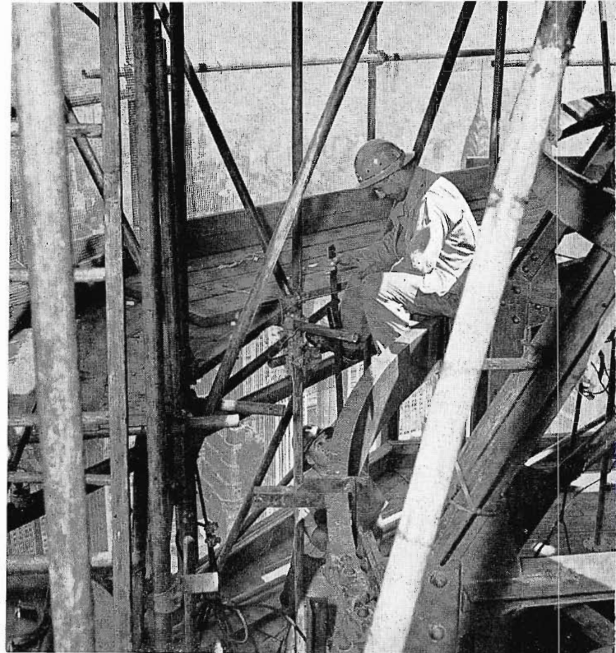
2 A three-story scaffold erected atop the Empire State building was necessary to provide adequate working space. Here, steel workers are shown completing the top working level, 1300 feet above the street level.
