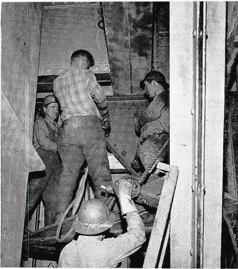
4 Here at the 96th floor, American Bridge Company steel workers are fastening new steel reinforcements to provide additional strength to accommodate increased activity, loads overhead, and the future 217-foot tower.
