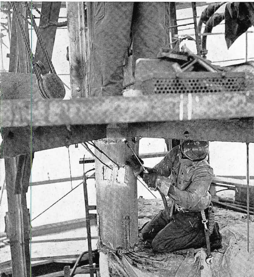
7 Section-by-section the old supporting pole was "burned-away" by the use of acetylene torches. Note that cable and pulley rigging is attached to the 400-pound section for safely lifting and "lowering-away".
